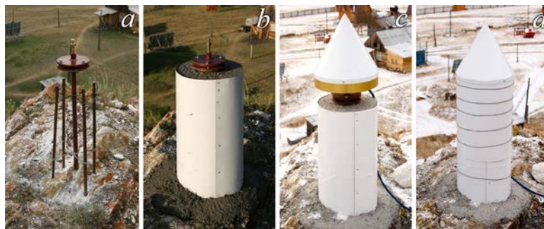
Figure 3. Stages of installation of a GNSS antenna on a bedrock base at the observation station UZUR (a–b)
